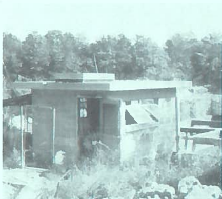
The old, delapidated water treatment plant in Dustin was built in the 30s when most work at the facility was done by hand.
